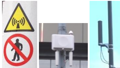
Cells intended for 5G may have ‘Radio Frequency Hazard’ stickers, high up
